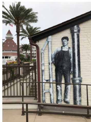
Exterior entry panels mounted to new sub-frame attached to existing brick wall.
